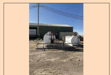
Fuel Tanks—1,000 Gal Gasoline, 2,500 Gal Diesel
