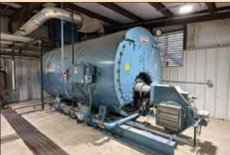
400 HP Superior Boiler
