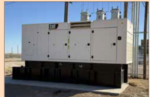
750KW CAT Generator
