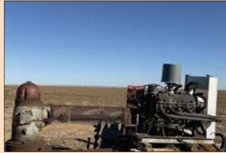
Water Well Motor and Turbine Pump
