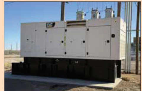
750KW CAT Generator
