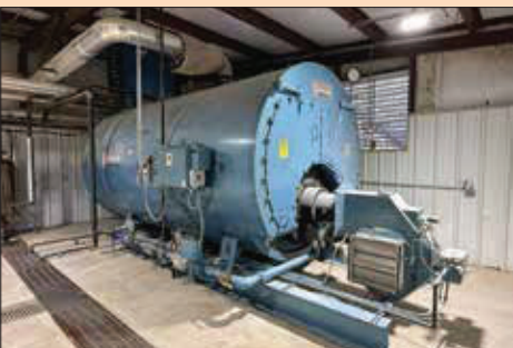
400 HP Superior Boiler
