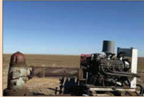
Water Well Motor and Turbine Pump
